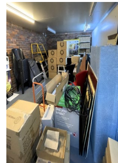
Inadequate storage to the rear of the photographic gallery
